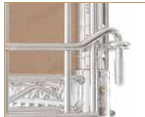
Protective cover on exposed wire ends.
